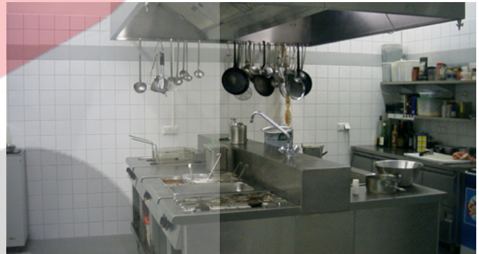
Filter monitoring in kitchens
